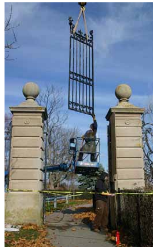
One of the Cliff Walk gates at The Breakers is removed. Photo by Andrea Carneiro
